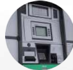
PETROL PUMP AND O.P.T
