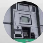
PETROL PUMP AND O.P.T
